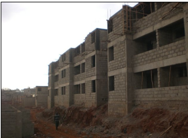
Fig. 9: KENSUP Phase 2 apartment blocks in Soweto East under construction, Kibera, photo by Lene Le Roux, September 2012.
