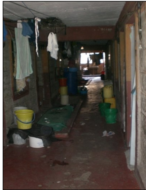
Fig. 14: Dark, damp corridor between units in a Huruma tenement building, photo by Lene Le Roux, September 2012.
