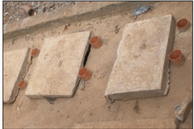
Fig. 6: Methane storage containers underground with ventilation pipes located next to bio-centre in Kibera, photo by Lene Le Roux, September 2012.
